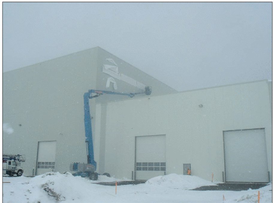
Installation was a serious challenge due to the 70 foot height—and the -17°C weather.
